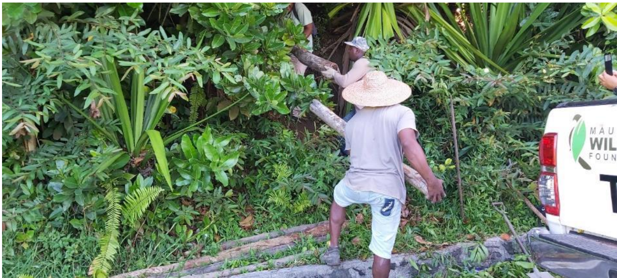
Plate 19. MWF staff, GMNR Restoration labourers and villagers from Thammes helped transport materials to the site.
